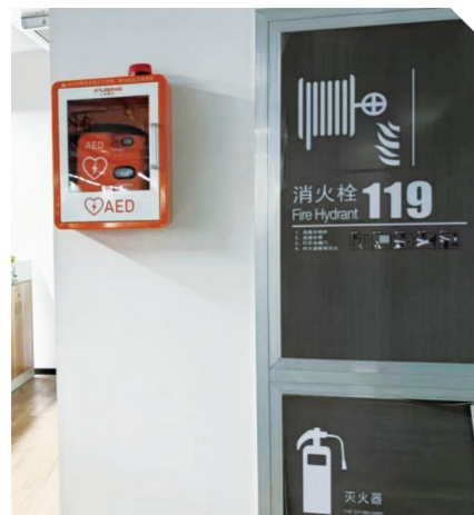
Equipping the workplace with Automated External Defibrillators (AEDs) and fire-fighting equipment
