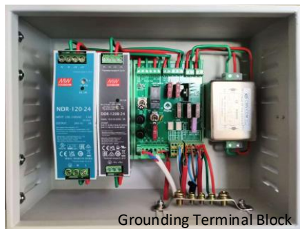
Grounding Terminal of Power Unit
